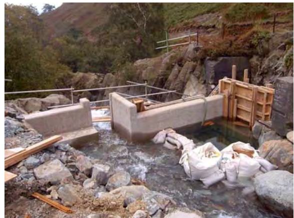
Construction of the new dam at the top of Church Beck Gorge.
