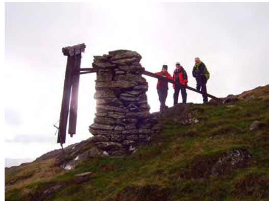
Pylon No 7. The wooden pylon has slipped off its base, but is still supported by its braces.
