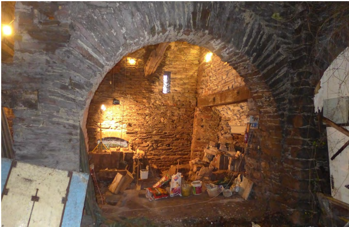
View of Blowing Chamber from adjoin workshop showing large arch for machinery access
