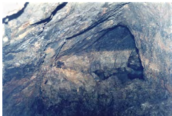
Near the collapse.
