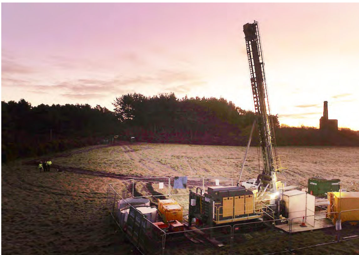
A photograph of the trial equipment installed to extract geothermal water samples from the granite rock deep below the surface at United Downs, Cornwall to assess the concentration of lithium present in the water.
