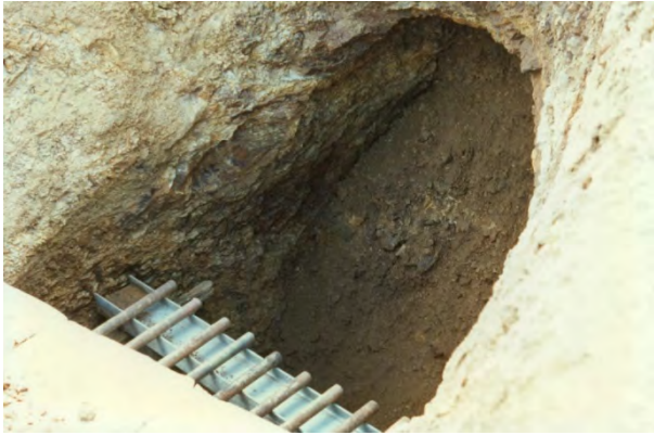
Ready to drive into the collapsed ground.
