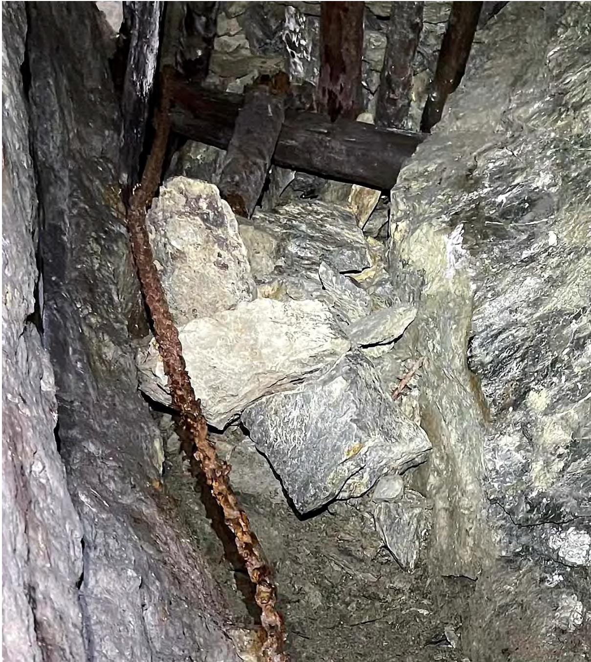
The rocks still remaining on the underside of the blockage.
