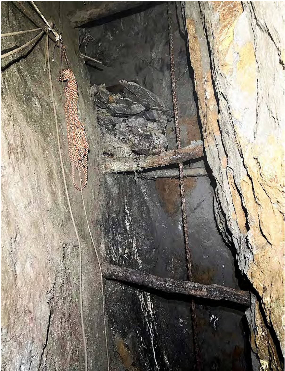
You can see the chain is still going down through the collapse.
